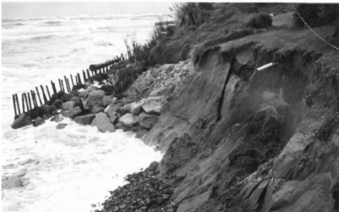
Plate 1 Erosion and loss of residential property at the southern end of Wainui Beach, Gisborne, 23 July 1992.
