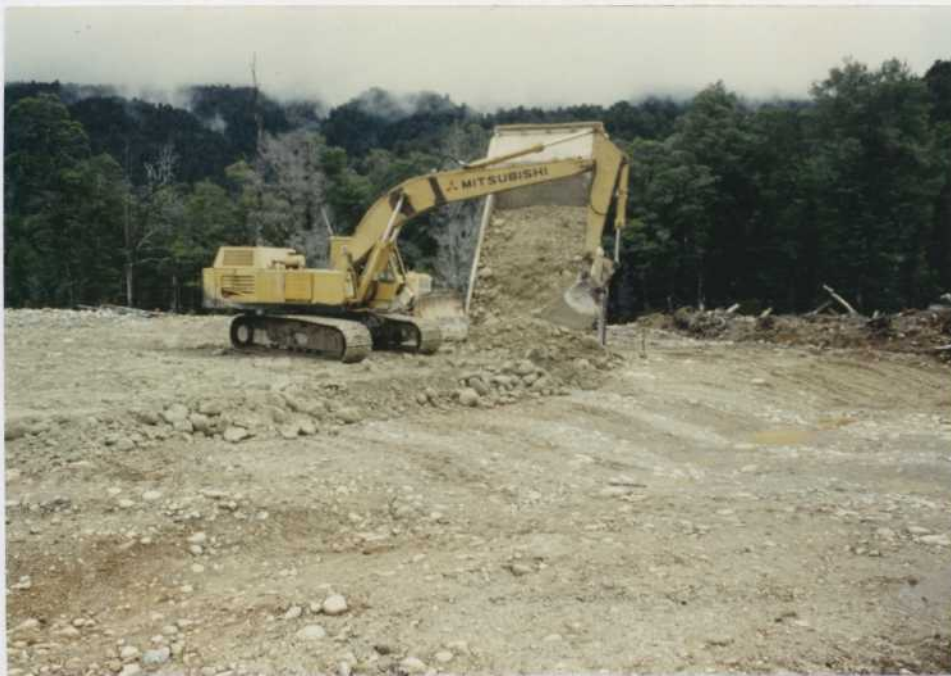
FIGURE 5. CONSTRUCTION OF THE GRAVEL PLATFORM FOR THE "GRAVELS TO THE SURFACE" TREATMENT.
