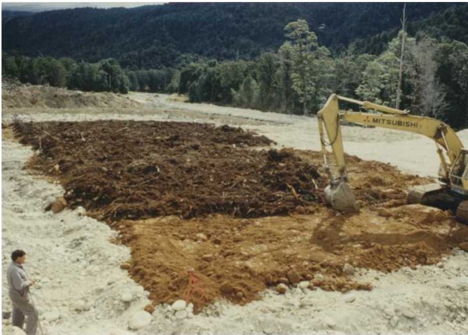
FIGURE 10. CONSTRUCTING THE ORIGINAL SOIL PROFILE PLOTS. THE "GRAVELS TO THE SURFACE" PLOTS ARE IMMEDIATELY BEHIND THE EXCAVATOR. THE MIXED SOIL REPLACEMENT PLOTS ARE IN THE BACKGROUND. THE ISOLATING OPEN DRAIN IS ALSO VISIBLE ALONG THE LEFT SIDE OF THE PHOTO.
