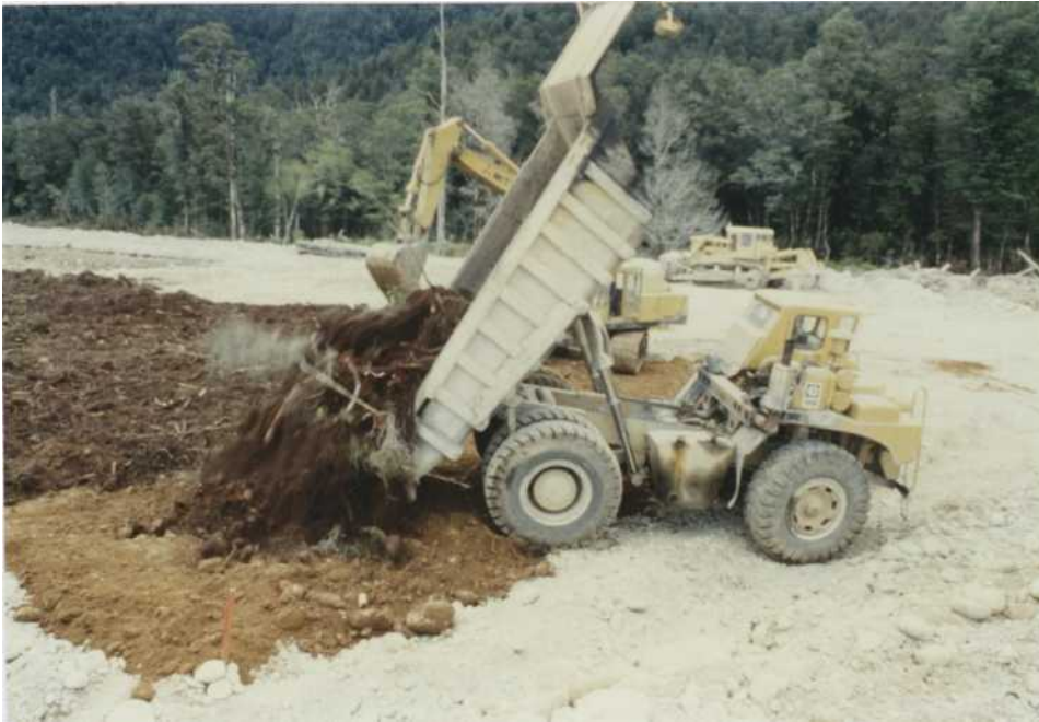
FIGURE 9. PLACING TOPSOIL AND ORGANIC MATERIALS OVER SUBSOIL BEFORE SPREADING WITH HYDRAULIC EXCAVATOR.
