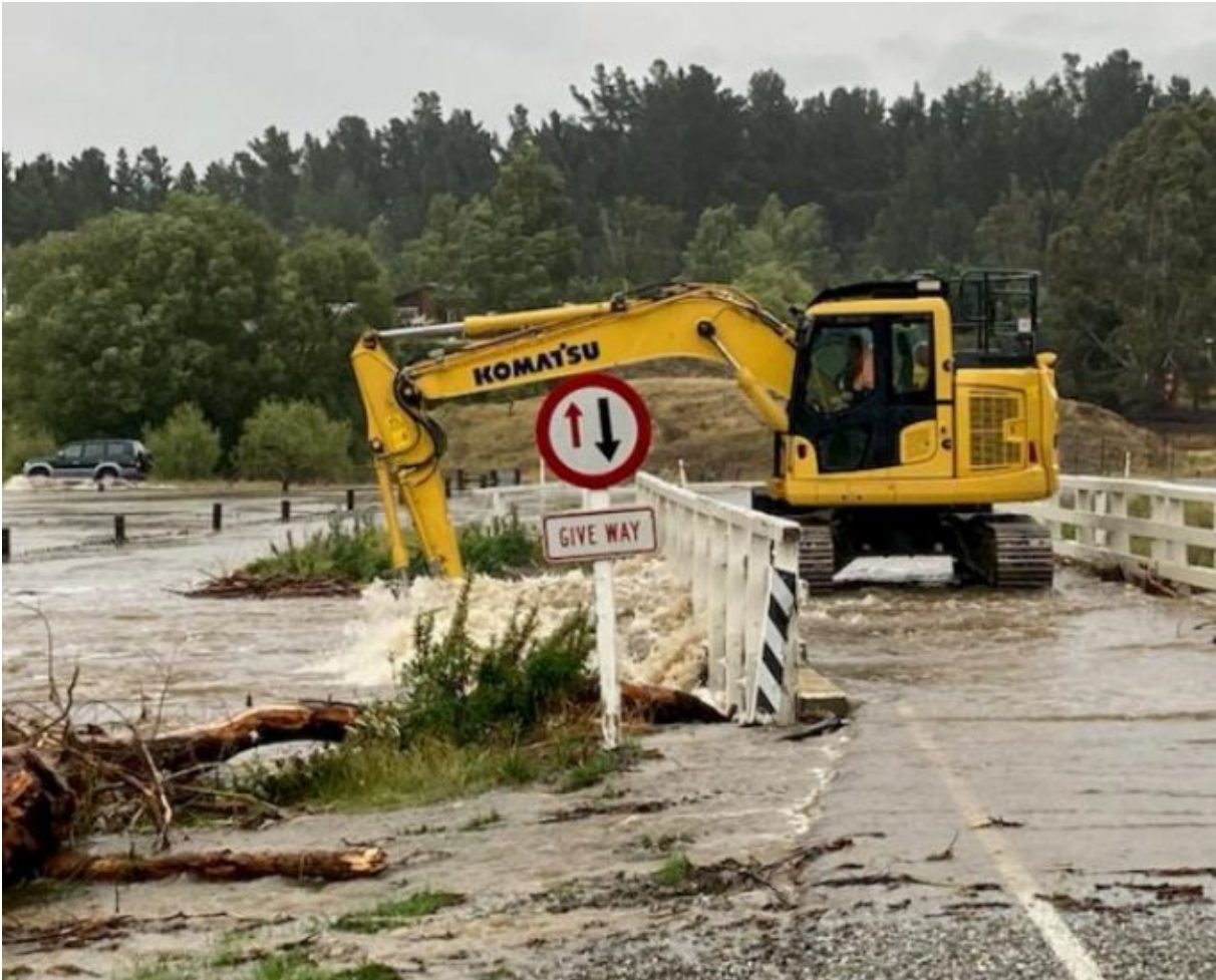
Figure 4-9 Patearoa township bridge being cleared of debris after flooding in the Mānīatoto in January 2021 (Source: Central Otago District Council/Fulton Hogan/Otago Daily Times)
