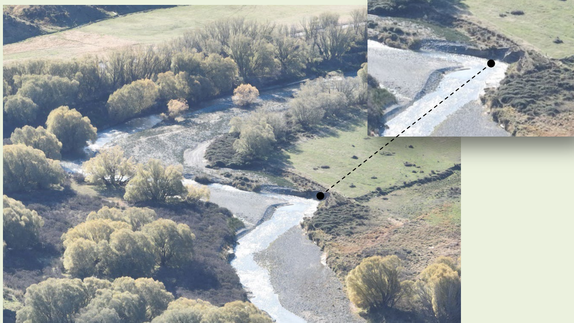
Bank erosion on the true left bank of the Kyeburn at Scott Lane (Source: GHC)
