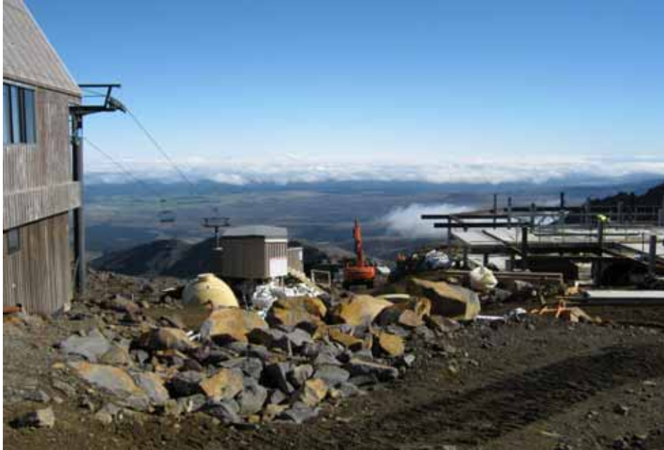
Site inspection of the new Knoll Ridge Café, Mount Ruapehu Photo: Jo Hood
