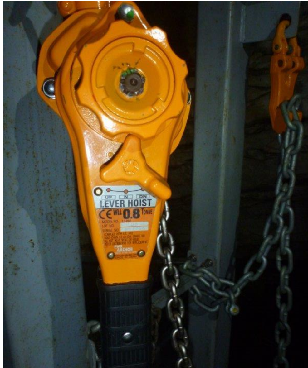
Figure 60. Photo of lever hoist used to raise and lower caves dam
