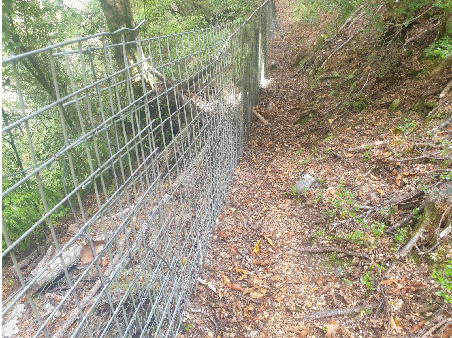
Figure 70. Photo of debris catch protection structures incl monitoring rock fall risks
