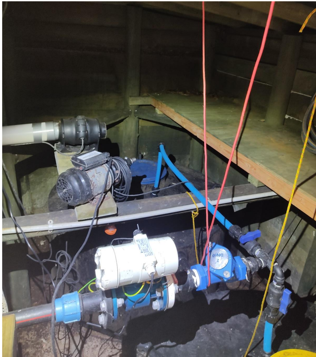
Figure 30. Photo of the interior of the wastewater treatment plant pumphouse bunker with pump well 1 and 2.
