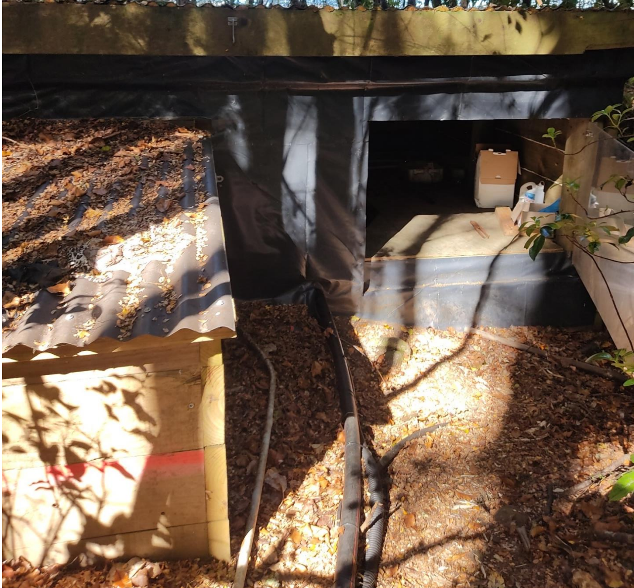
Figure 29. Photo of exterior of wastewater treatment plant pumphouse bunker (the tanks used to collect the liquid overflow from septic tank prior to pumping to AES disposal field)
