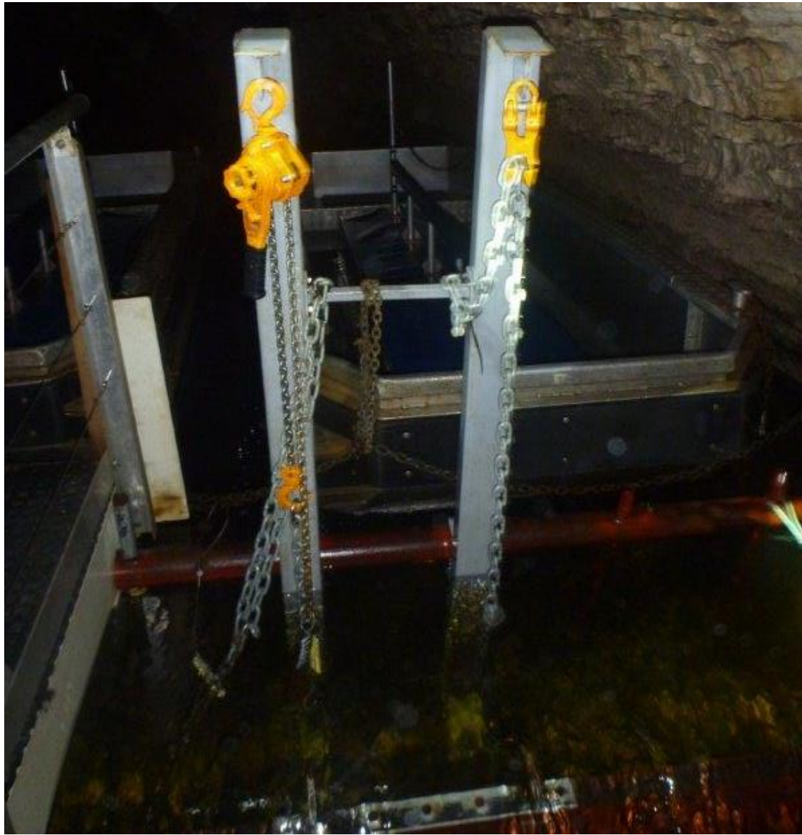
Figure 59. Photo of hoist system used to raise and lower caves dam
