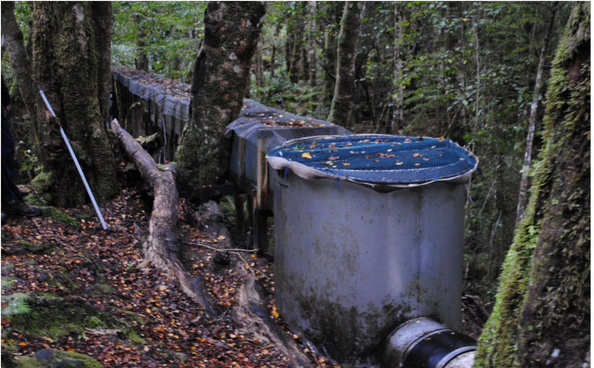
Figure 33. Photo of surge tank and the start of the hydro pipeline
