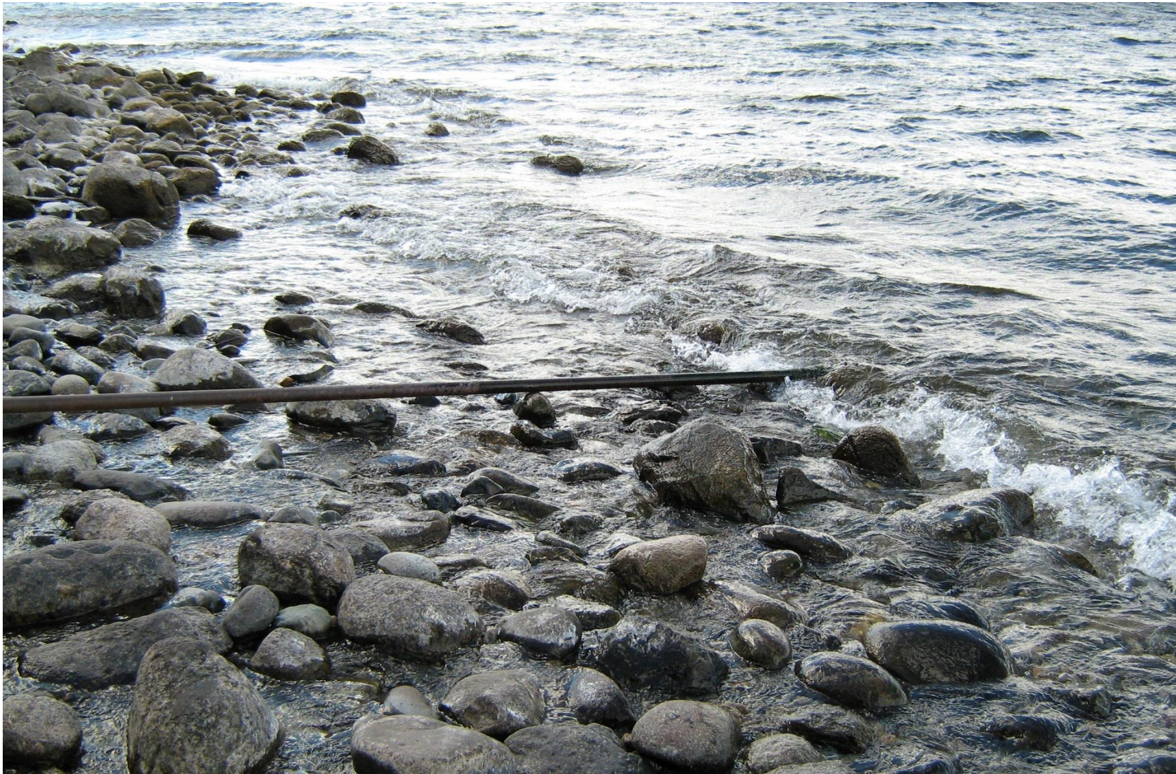
Figure 45. Photo of pipeline for lake water take when unnamed stream is low
