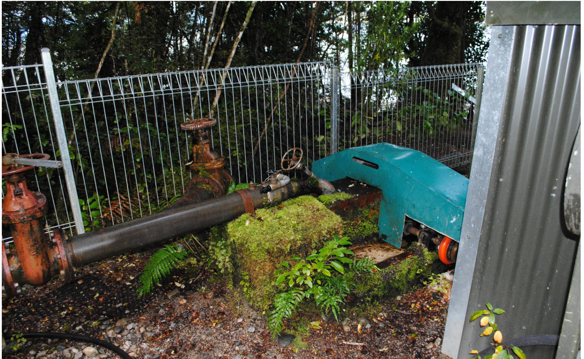
Figure 38. Photo of Hydro inside enclosure
