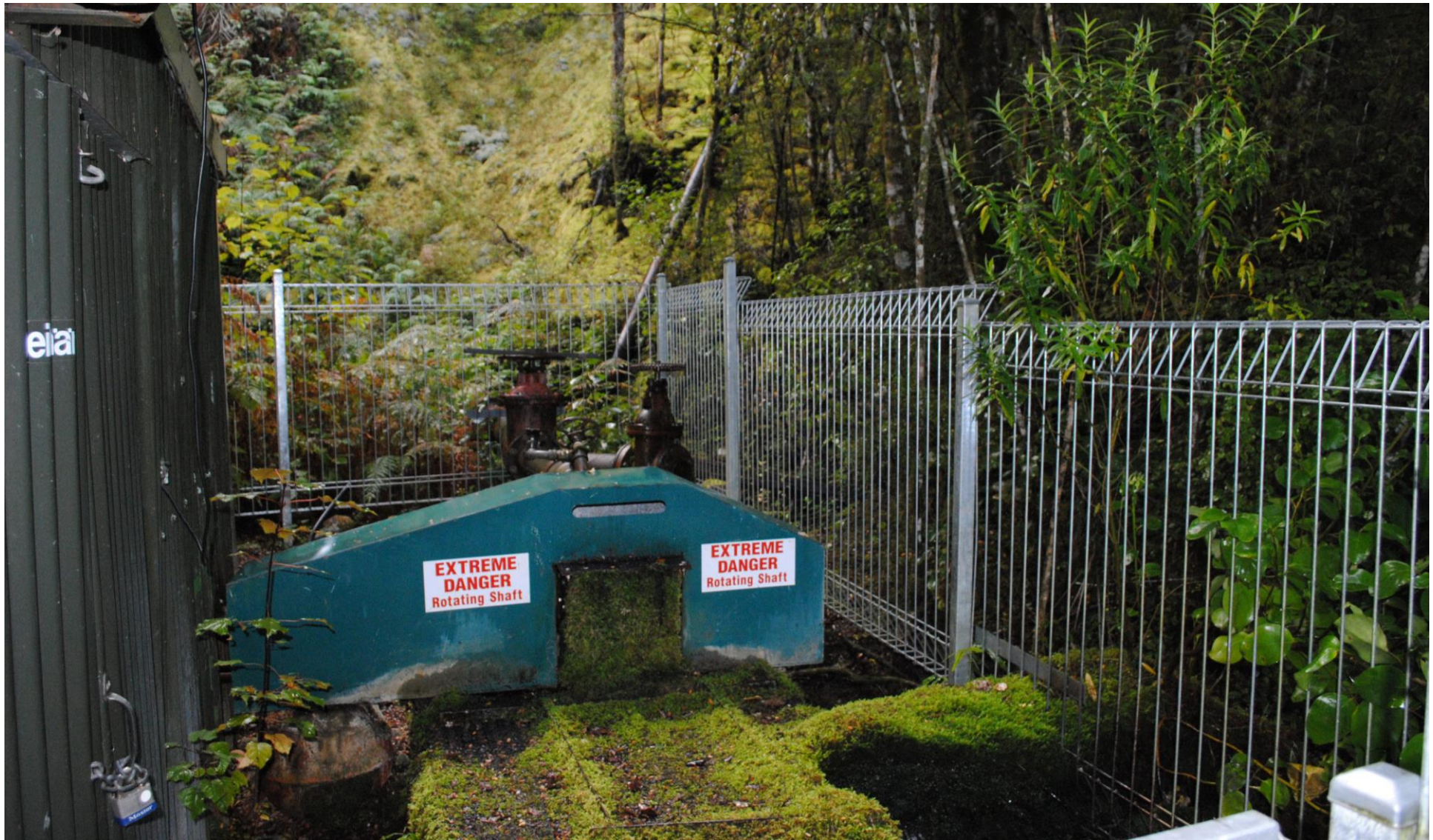
Figure 37. Hydro including its enclosure
