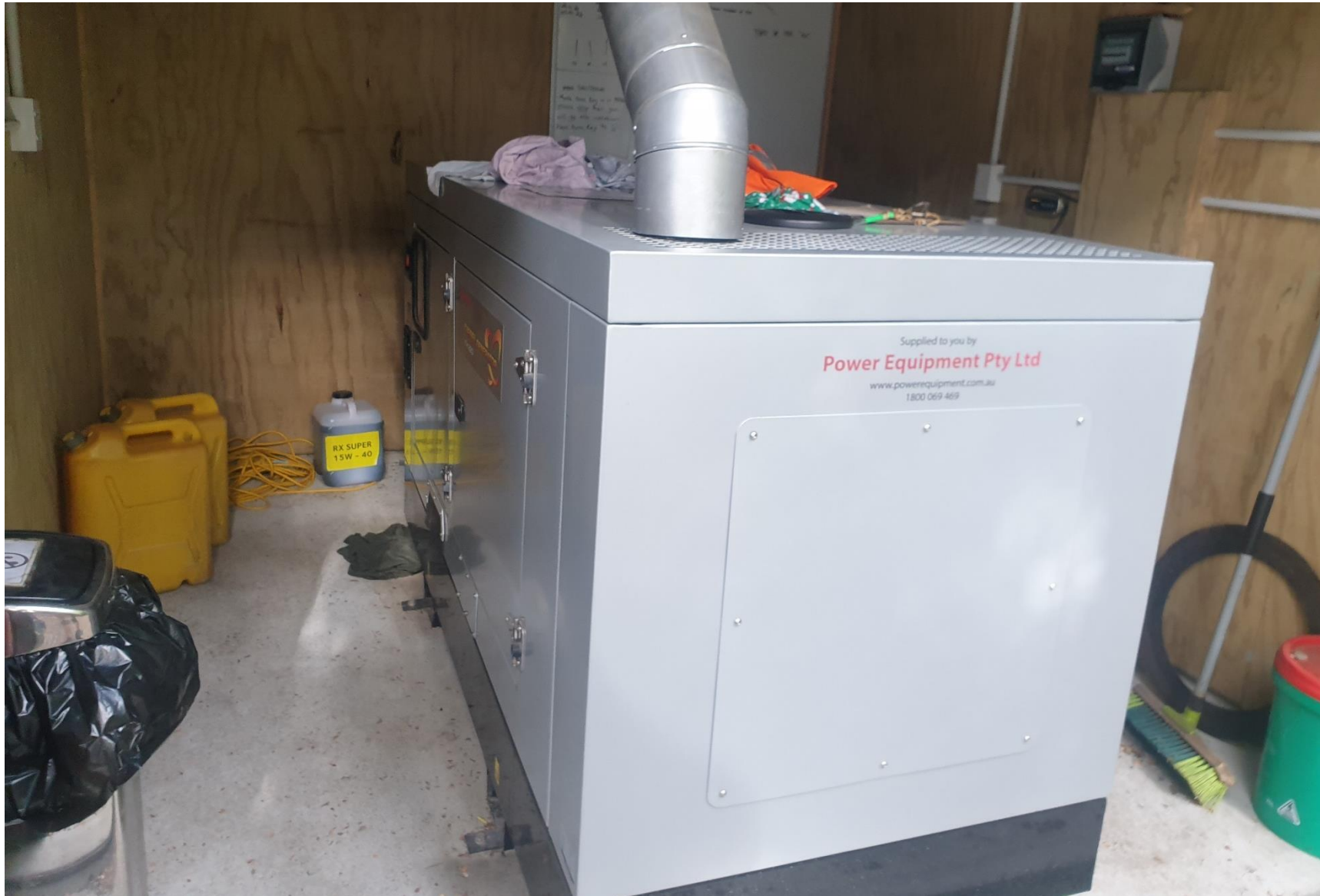
Figure 44. Photo of Yanmar generator
