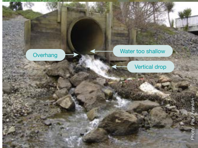
Captions (from top): A weir fish passage barrier in a waterway; a tide gate fish barrier in a waterway; a perched overhanging culvert fish barrier in a waterway.
