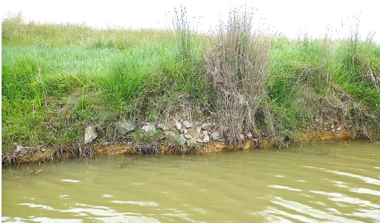
Figure 5: Western side of the Pungarehu Canal between the farm bridge and the Whangamarino wetland has a thick layer of gravel and stones. This material was not present on the Eastern side of the canal.
