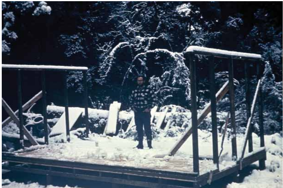
The frame of Lake Te Au Hut, Murchison Mountains 1963. Max Evans, local field officer pictured. This hut was later moved after the site was found to be flood prone.
