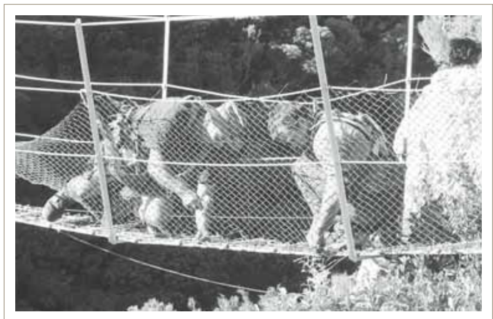
DOC rangers, Ricky Croft (left) and Cameron Jones tie new nylon safety netting onto the bridge over the Harman River, 22 metres above the water.
