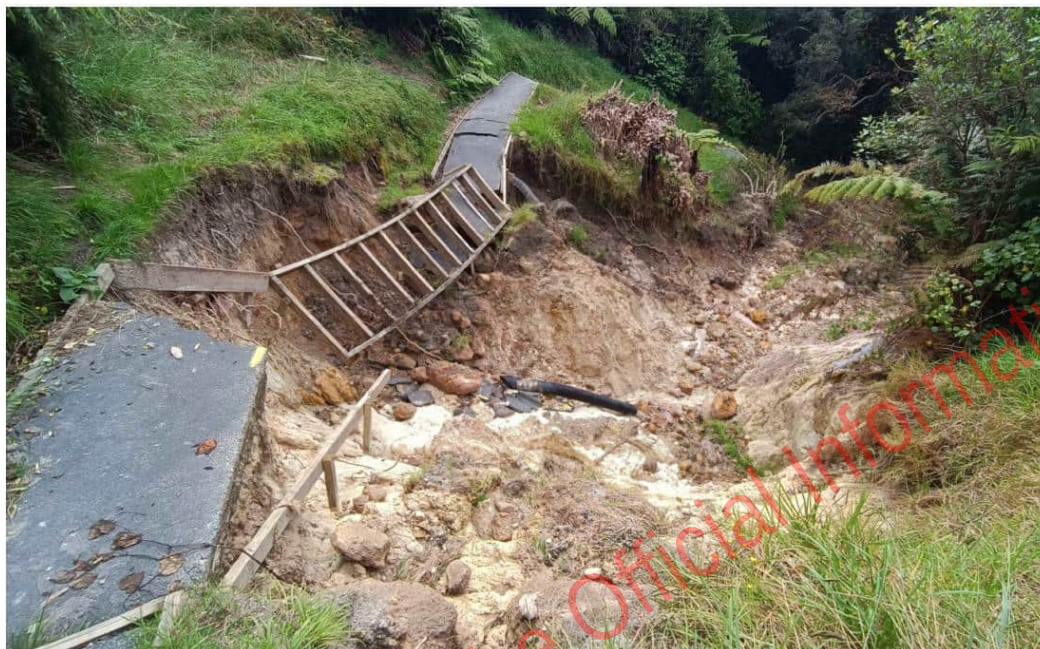
Figure 2.1: Cathedral Cove lower track landslide damage.
