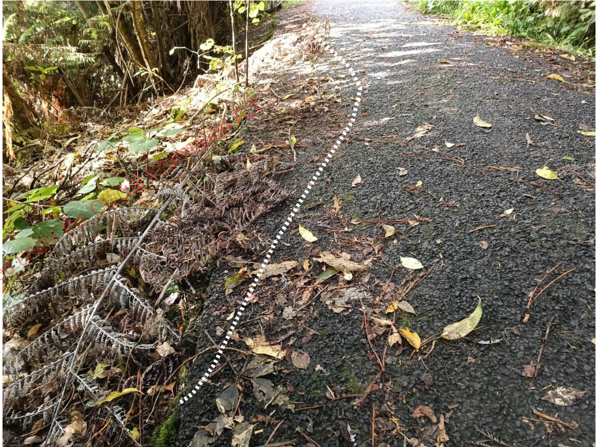
Feature 194 - Tension crack. Newly observed in May 2024 visit. This event is difficult to see and likely to be historical.
