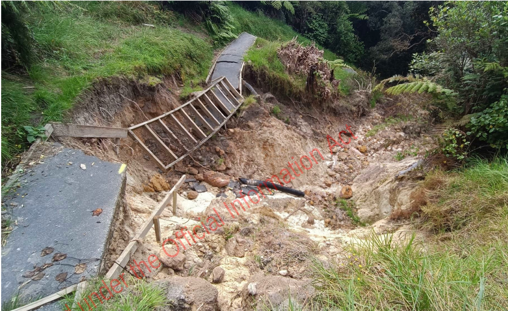
Figure 10.1 Cathedral Cove lower track landslide damage.
