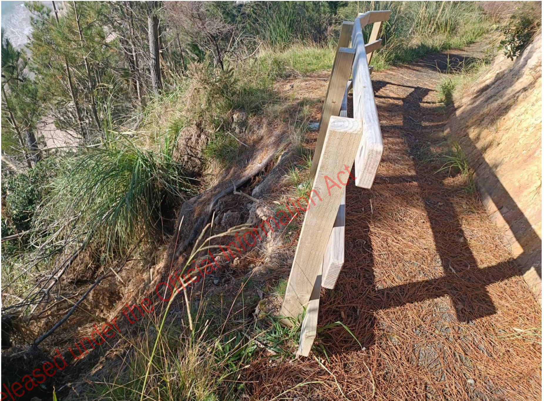
Figure C14 Landslide scarp close to Hahei Track
