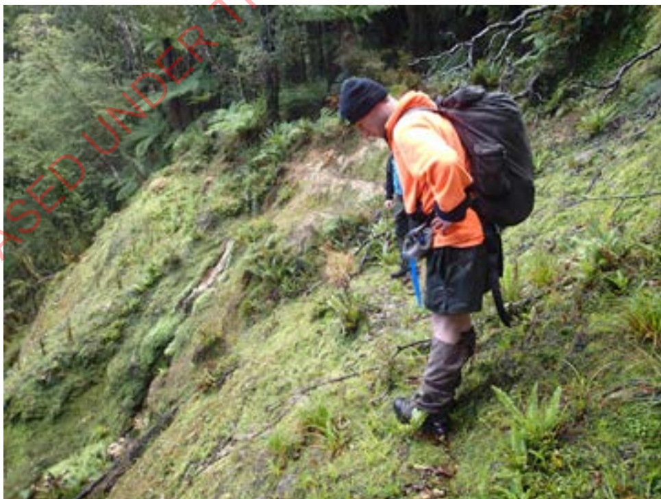
Figure 17. An area where the original line of the track has been destroyed by slips.
