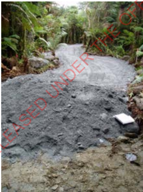
Figure 11: Stage Two - Stripping of organic matter and topsoil to stockpile for later use, and placement of basecourse.
