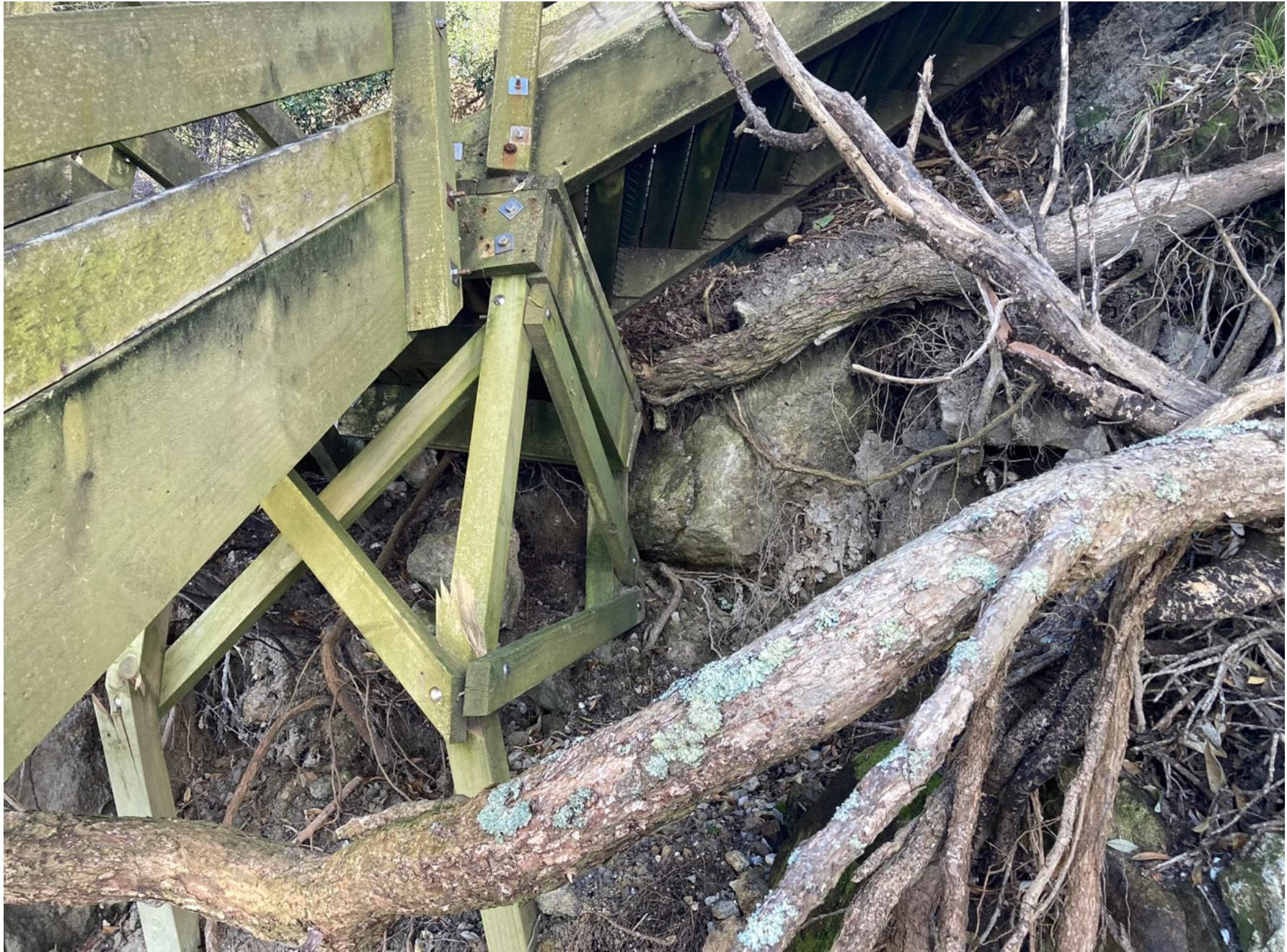
Figure C12 Gemstone Bay stair access damage and scour of loose boulders in slope.
