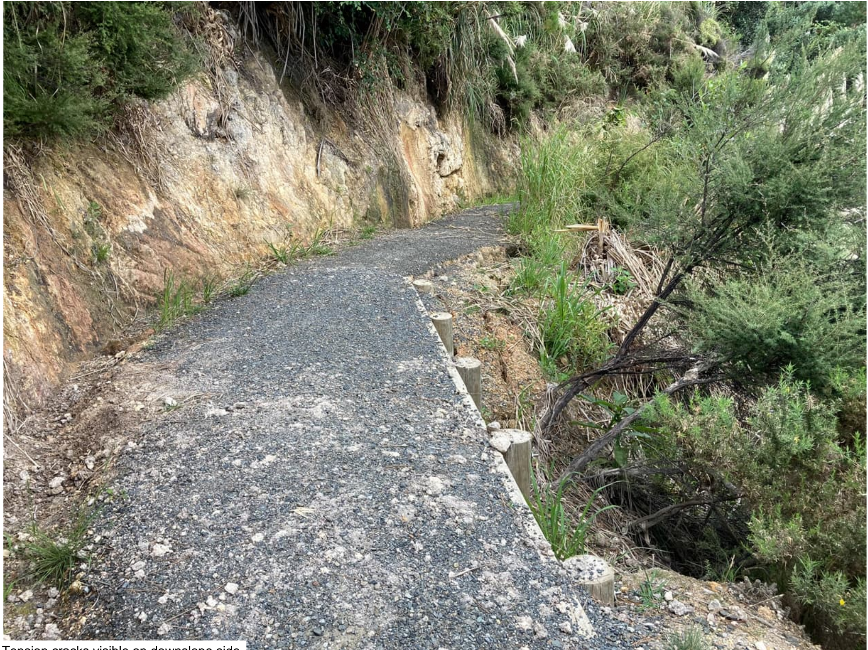
Figure C14 Tension cracks visible on downslope side of Hahei Track
