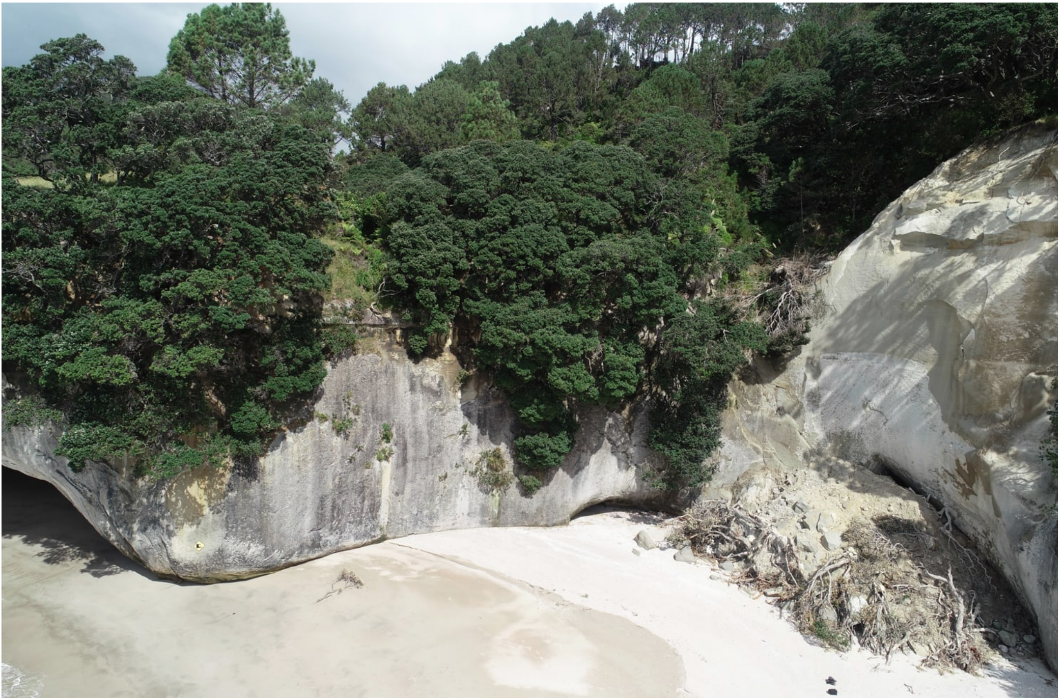
Figure C3 Recent and historical debris / talus at the toe of the coastal cliff on Cathedral Cove Beach
