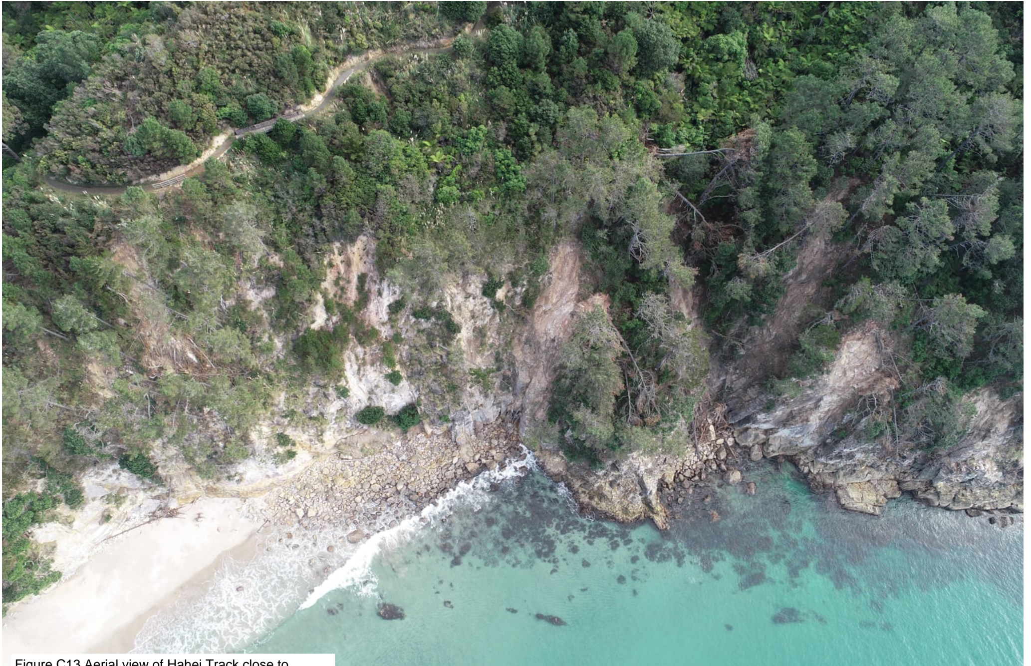
Figure C13 Aerial view of Hahei Track close to coastal cliff and recent landslides.
