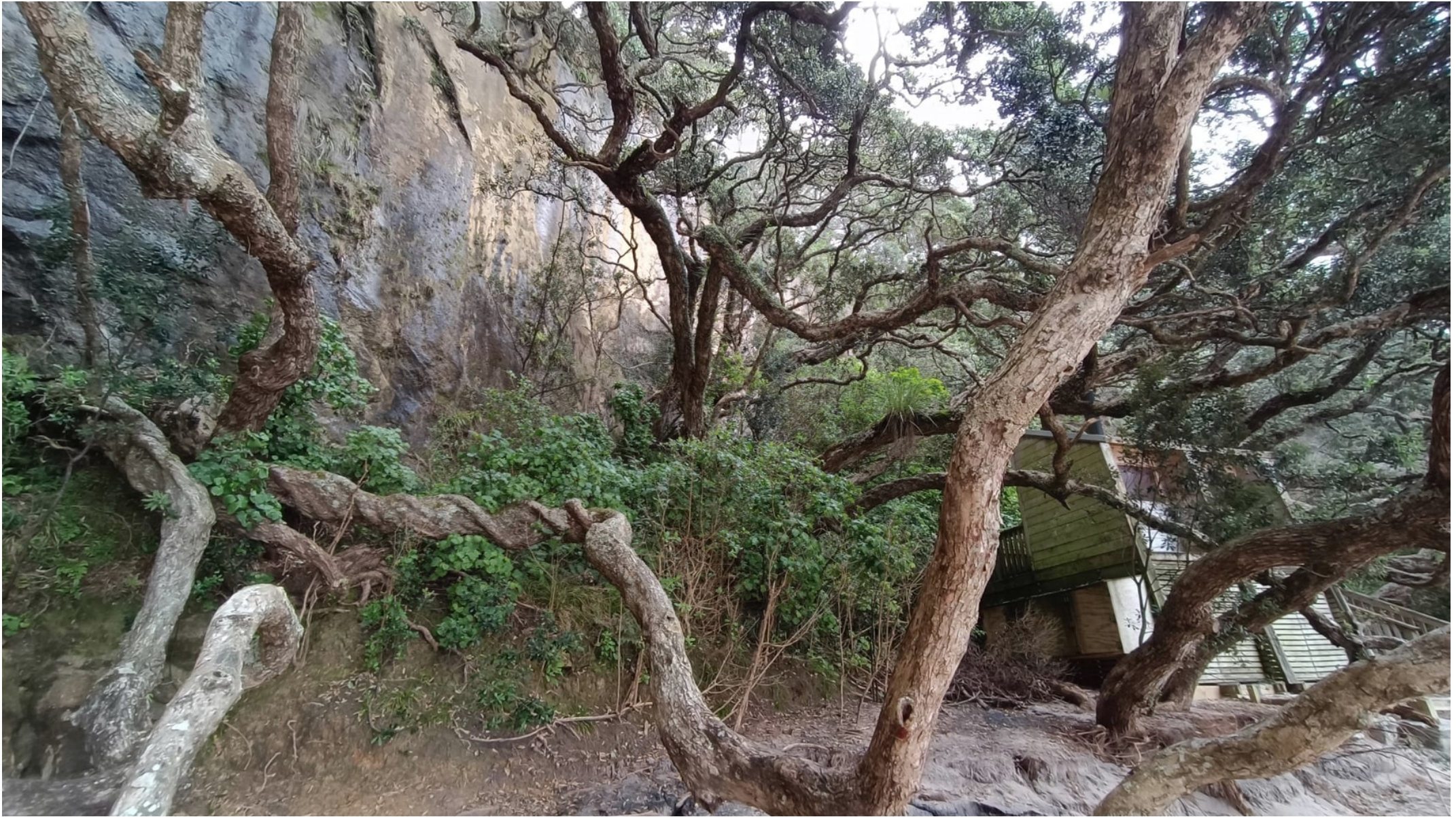
Figure C2 Historical debris / talus at the toe of the coastal cliff behind the existing toilet at Cathedral Cove Beach
