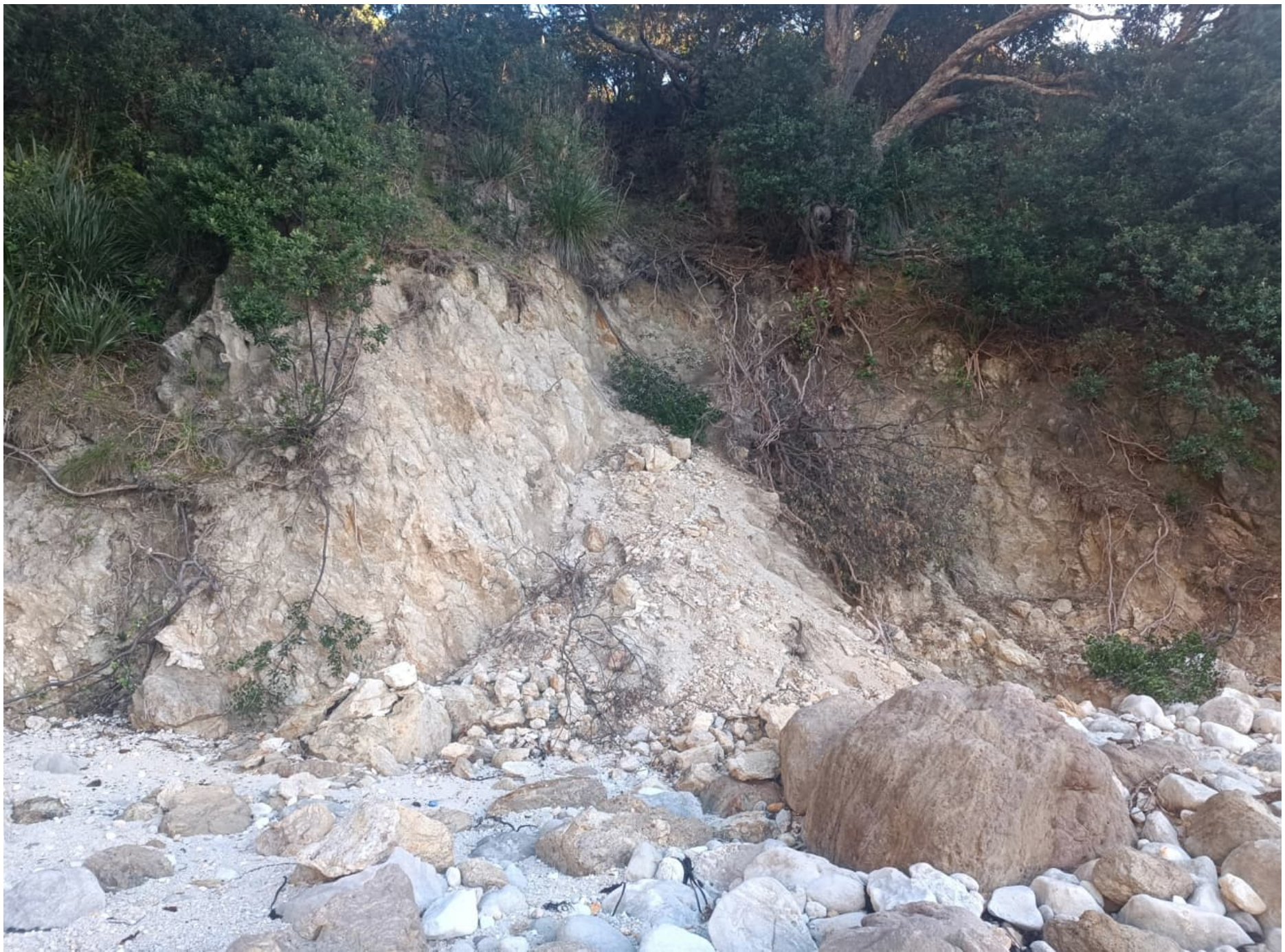
Figure C10 Rock and landslide debris at north end of Gemstone Bay
