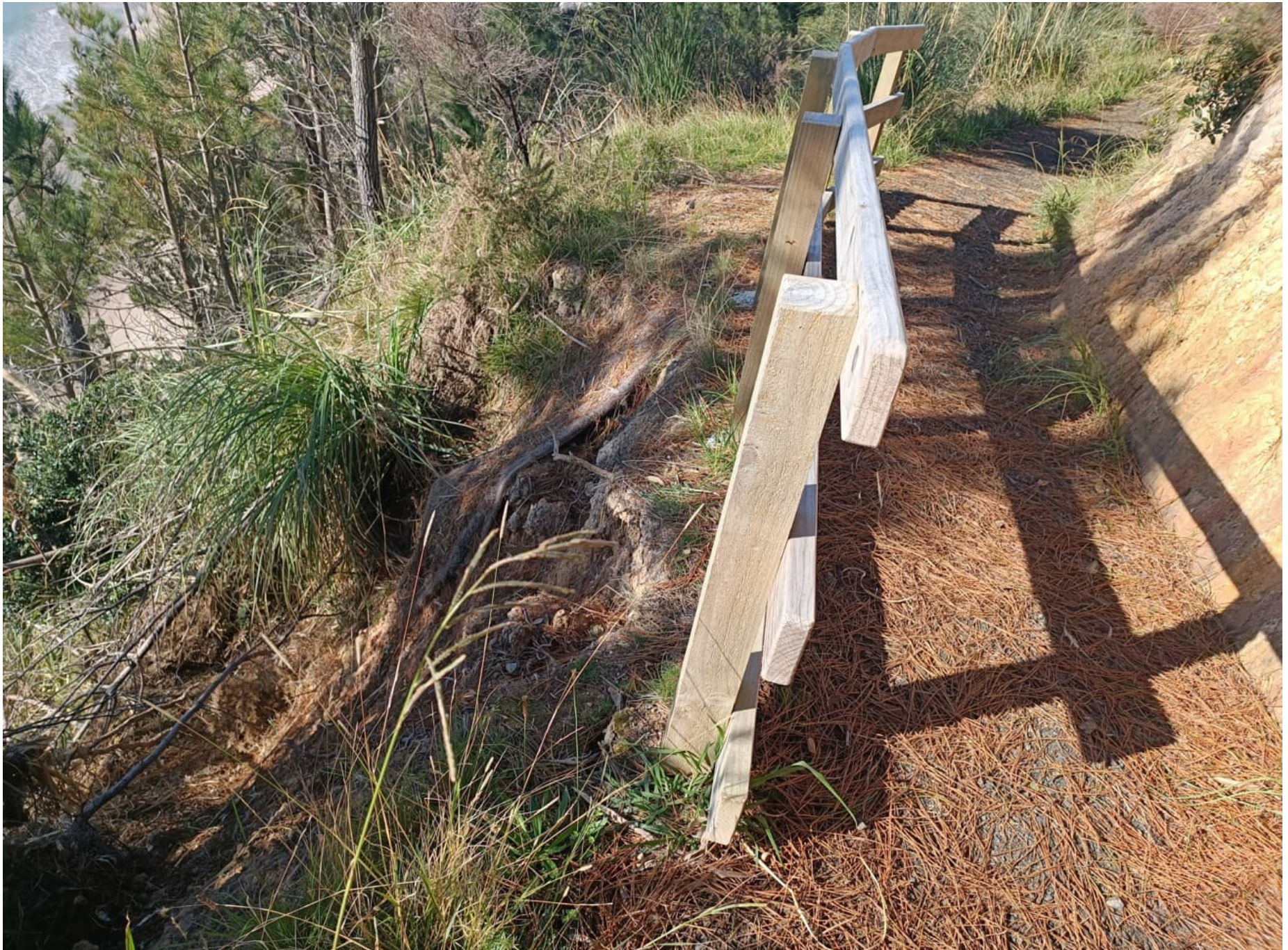
Figure C14 Landslide scarp close to Hahei Track
