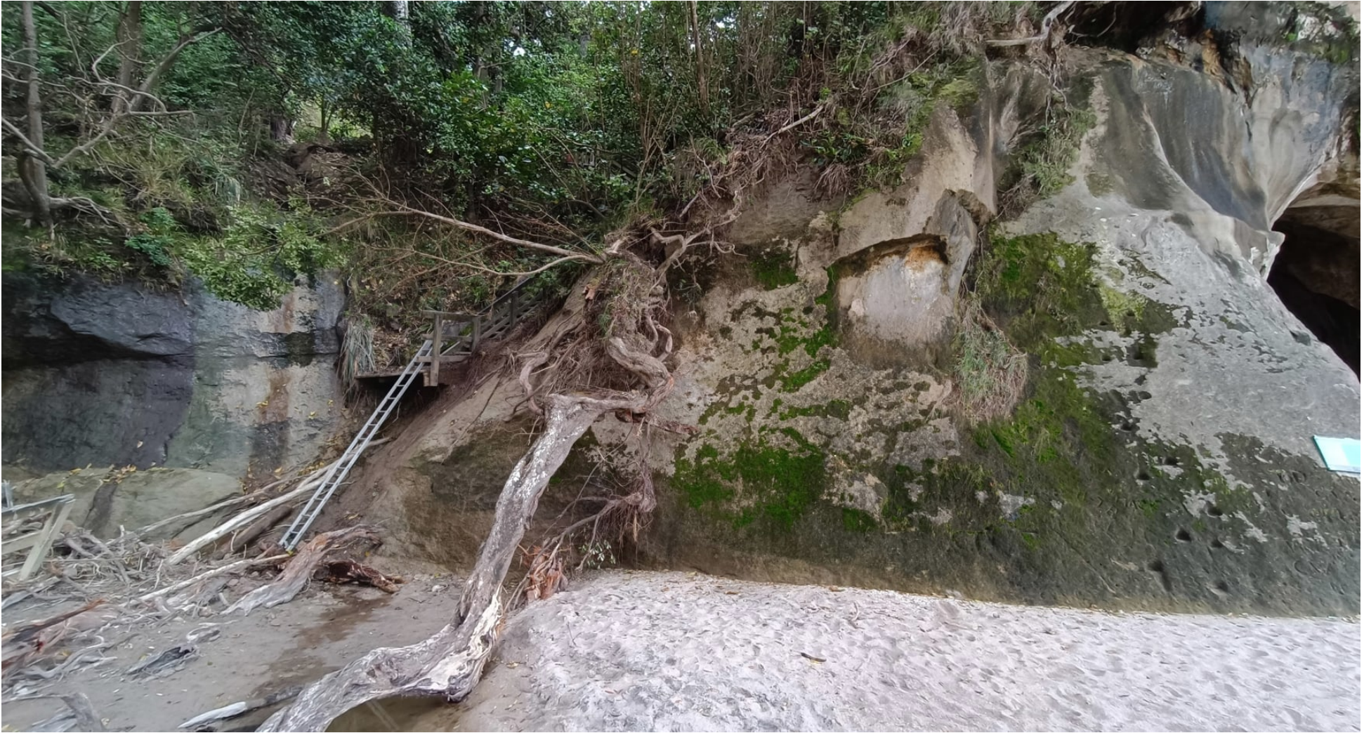
Figure C1 Damage to Cathedral Cove Access
