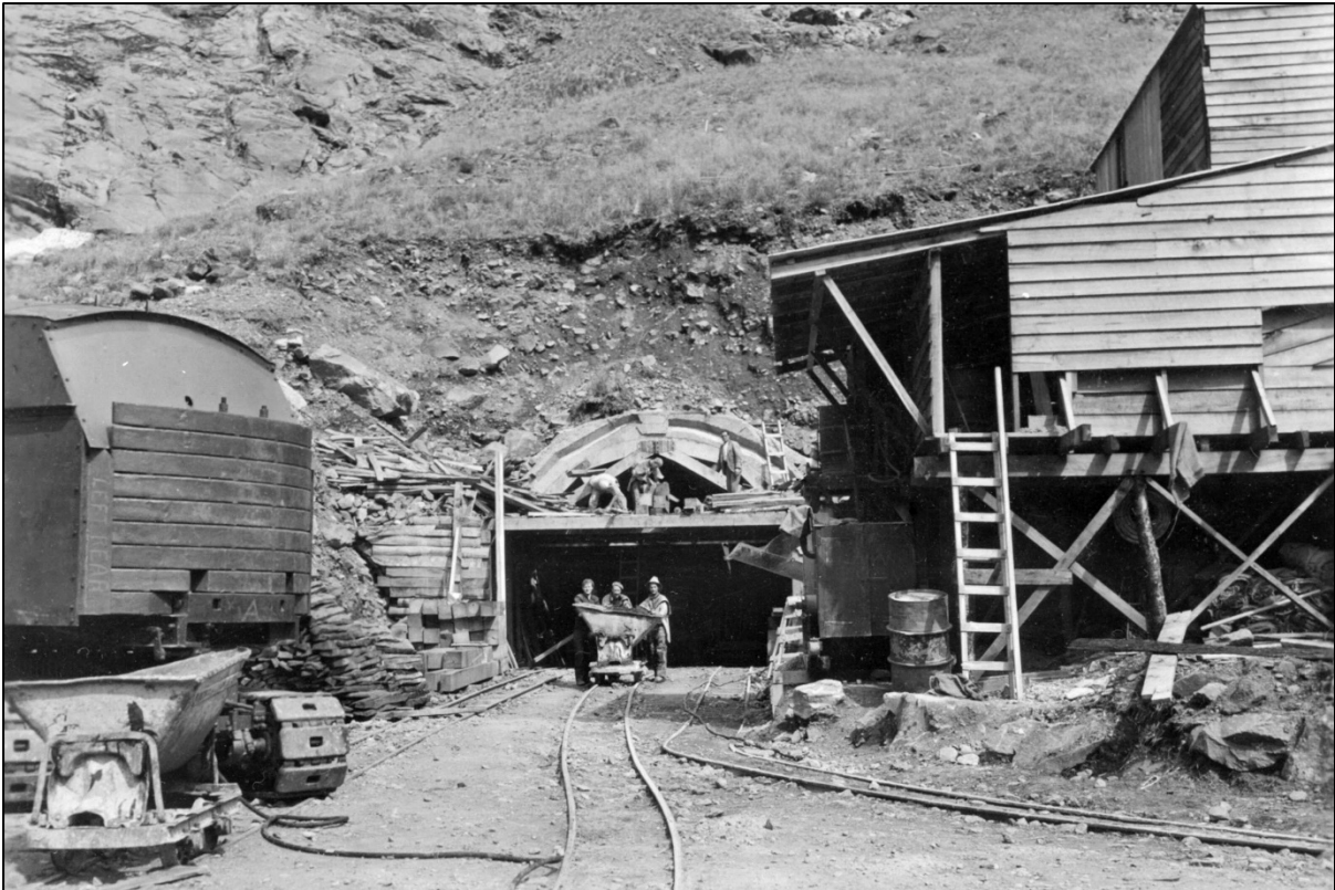
Figure 2. Constructing the eastern tunnel portal in 1936. 27 The original timber drill shed is on the right.
