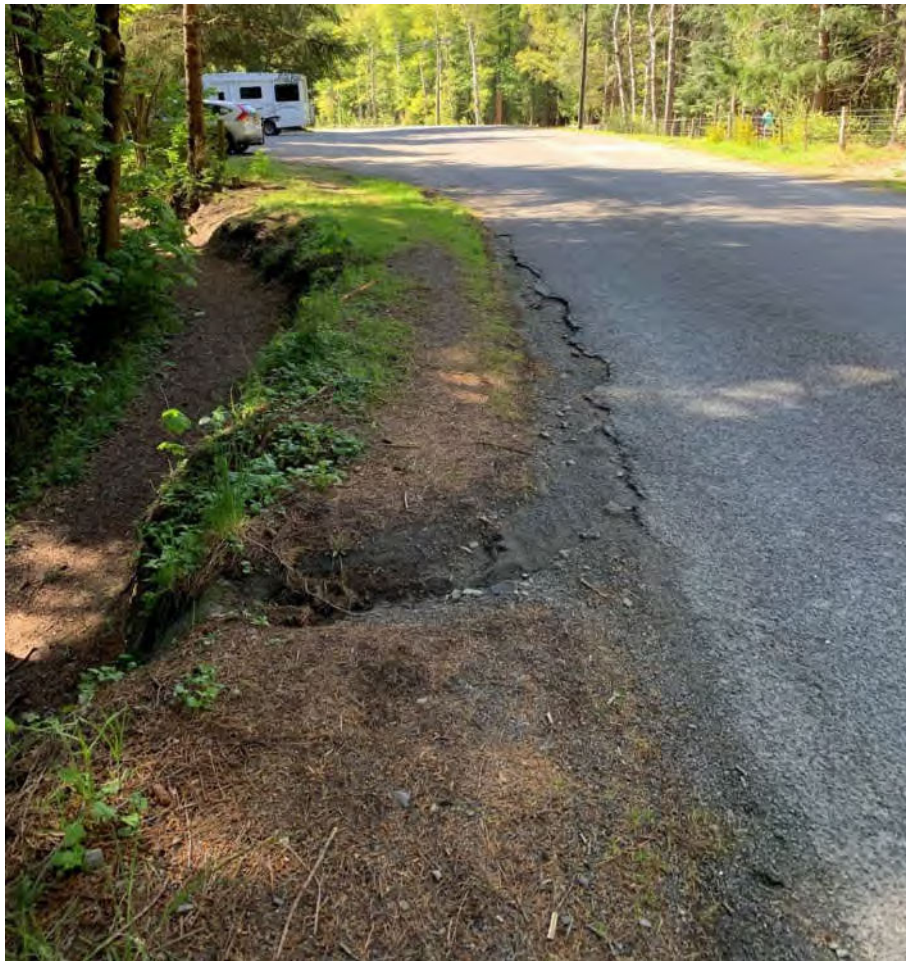
Photograph 12: Track Along the Edge of the Road Shows Potential Water Damage (Edge of Seal and Culvert Location)
