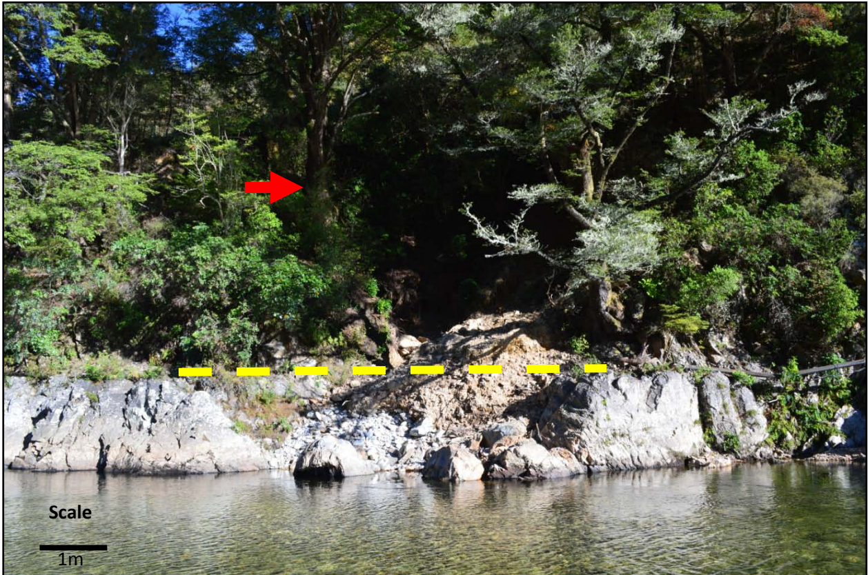
Figure 4. Photograph of the rock tunnel slip, taken from across the river, photo taken May 14 th , 2013. Yellow dashed line indicates the level where rip rap should be placed up to (atleast), based on the scour level on the slip toe from high flow. The red arrow points to a tree that is recommended to be removed.
