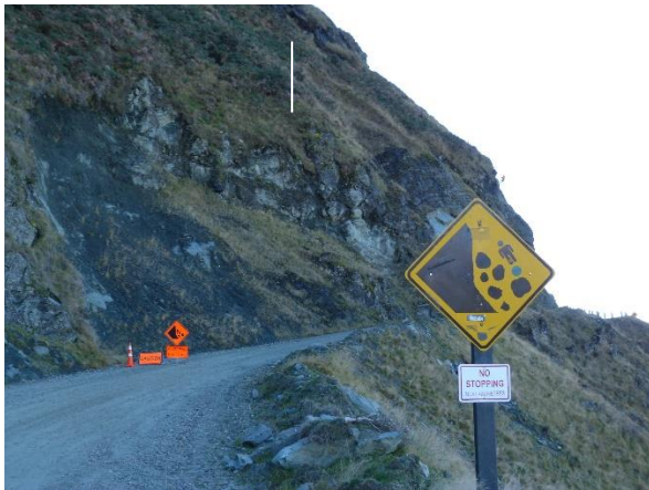
Photo 1 – new no stopping sign (uphill approach)
