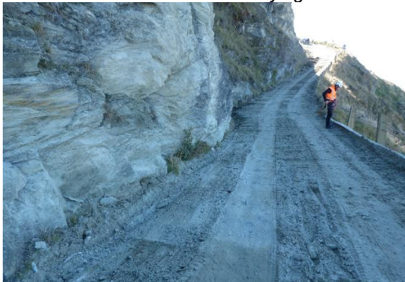
Photos 8 – Concrete Dish channel blocked
