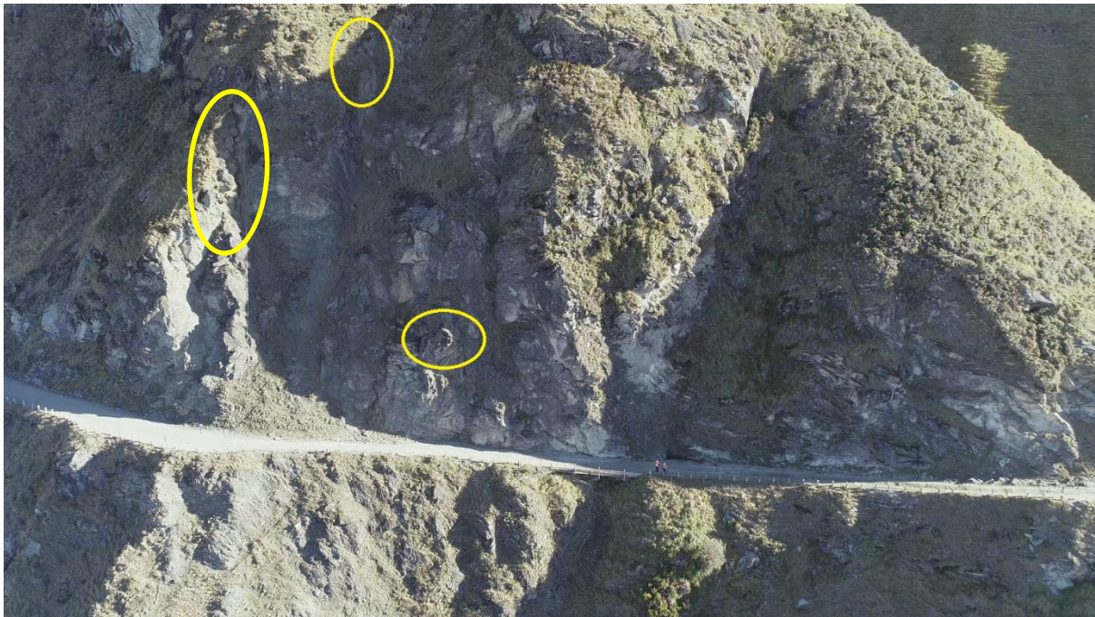
Photo 16 – Three particular areas to be monitored in 2018, also includes Grid reference A2 adjacent the measurement waratahs (far left circle on photo above)
